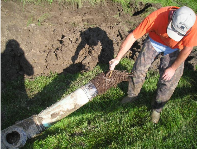
Figure 1. The section of plugged tile must be located and cut out from the system. These dense fibrous roots from a nearby tree entered through perforations in the tile and completely blocked water flow. The root wad grew so densely it filled the tile to the point the ribbings of the tile can be seen in the root wad that is being held.
