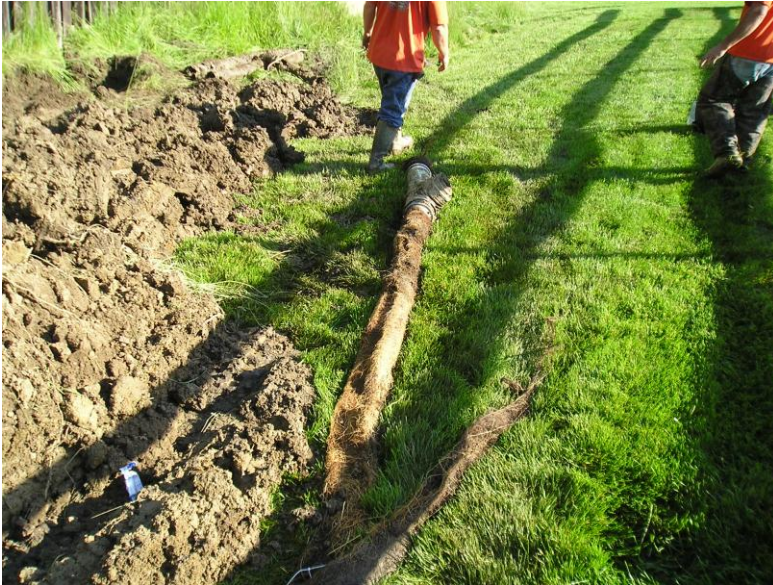
Figure 2. A lengthy section of 8 inch tile was plugged solid with roots. The roots originated from a large willow tree located more than 30 feet away from the buried drain. The plugged section, about 70 feet in length, was cut out and replaced with non-perforated pipe to prevent roots from entering again.
