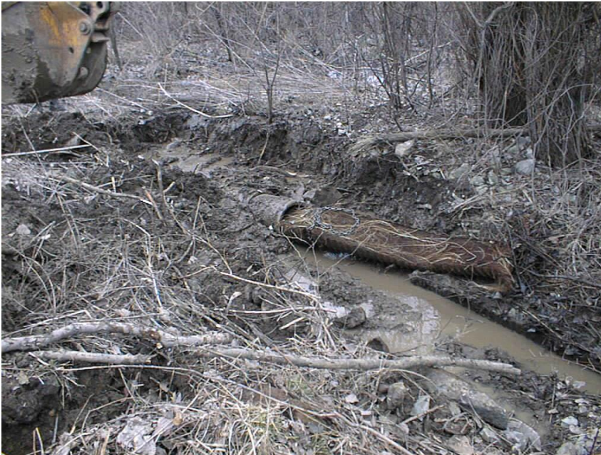
Figure 3. An example of a 15 inch drain tile completely plugged by tree roots. Tile drains as large as 30 inches in diameter have been completely plugged by tree roots
